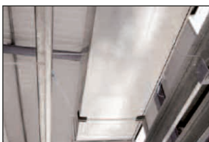
Square Air Ducts
