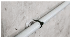
Flexible or rigid cable conduits with cable ties
